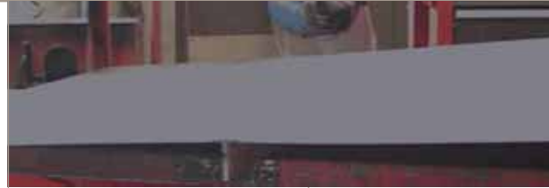
Twisted-buckled panel after welding
